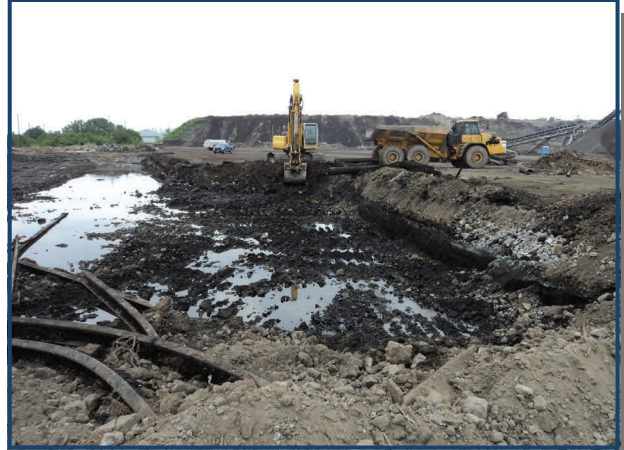
View of project area during construction. Materials excavated included steel slag, a deteriorating bioremediation system, and an abandoned railway.
