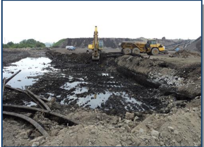
View of project area during construction. Excavated materials include steel slag, a deteriorating bioremediation system, and an abandoned railway.
