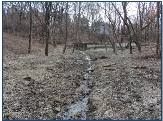
Existing natural basin that will be modified into a floodplain enhancement area.
