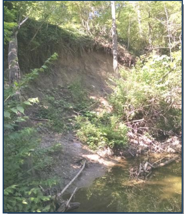
Lateral channel migration and non-cohesive soils have led to a steep, actively eroding streambank at this site. The top of the streambank is within 20 feet of the road.
