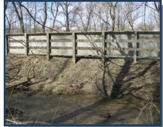
Pre-construction photo of eroding streambank at Glady Run, immediately adjacent to the Little Miami Scenic Trail bike path.
